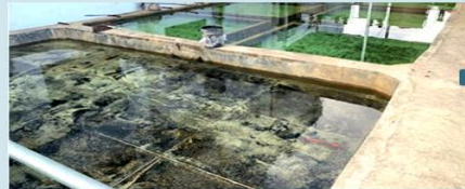
Biological Sedimentation Tank
